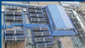
Qingdao Union Data Center
